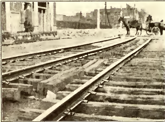
SPECIAL TIE PLATES IN ST. LOUIS TRACK
